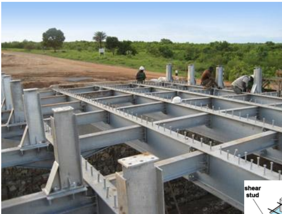
Figure 8: Composite Girders used in a steel bridge (left). Typical composite construction. (right).
